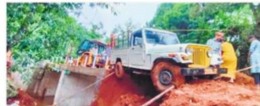
The newly-built bridge at Niduvale in Kalasa taluk which caved in
